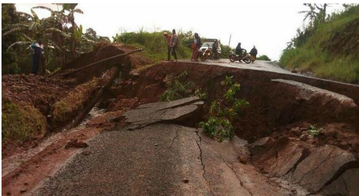
Figure 8-17: Calamitous state of roads in the North West.
