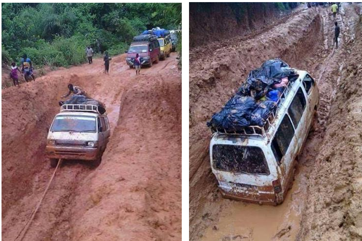
Figure 4-1: Deplorable condition of rural roads in the Western Highlands of Cameroon.
