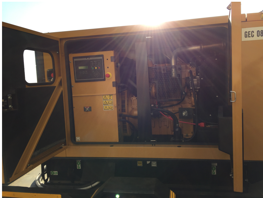
FIGURE 4.5: DE88E0 Catapillar diesel electric generator with 70 kW output.
