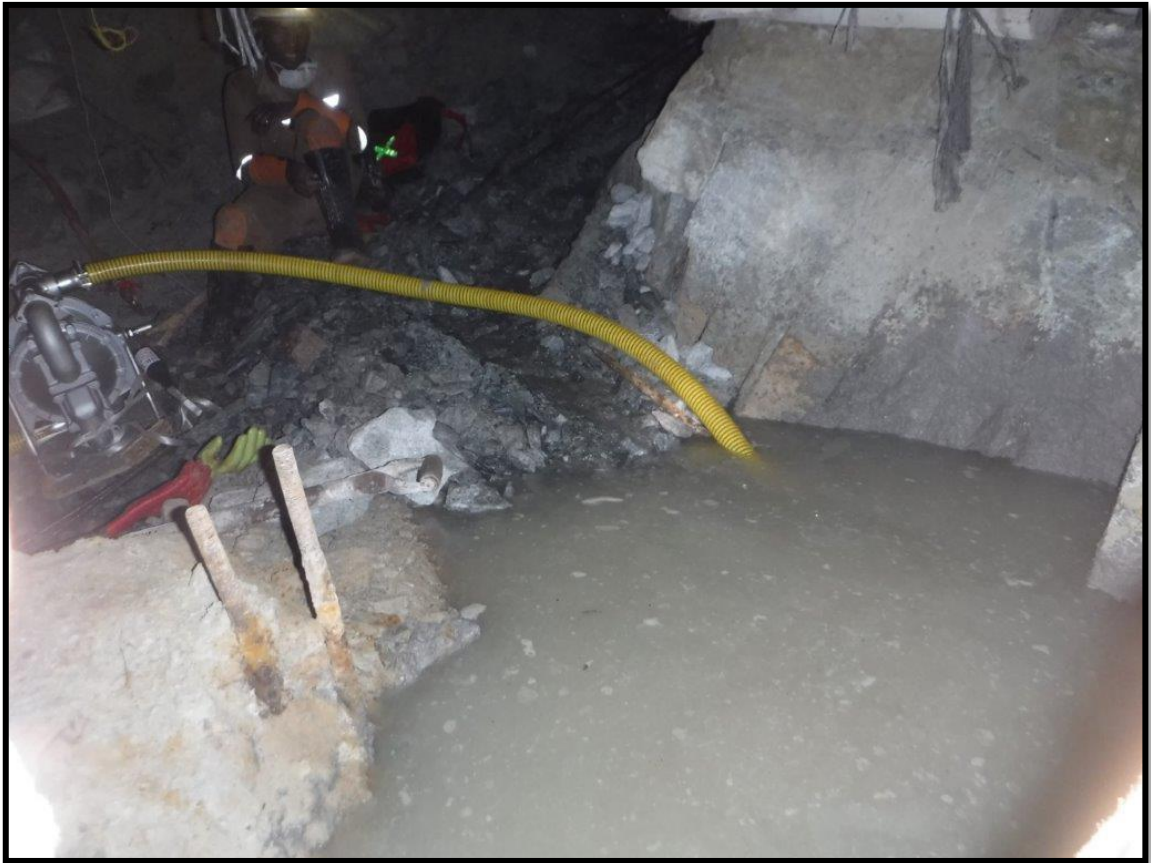
Figure 5-20: Centrifugal pump to pump water out of the stope (Botes, 2021)
