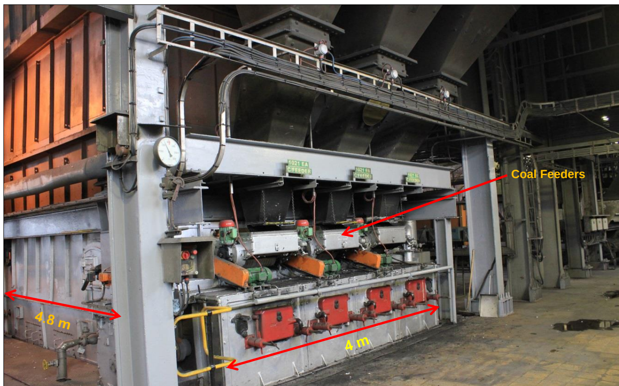
Figure 2.3A: Picture of Impala spreader stoker boiler unit No.5 showing furnace layout [photograph courtesy of Impala boiler archives]
