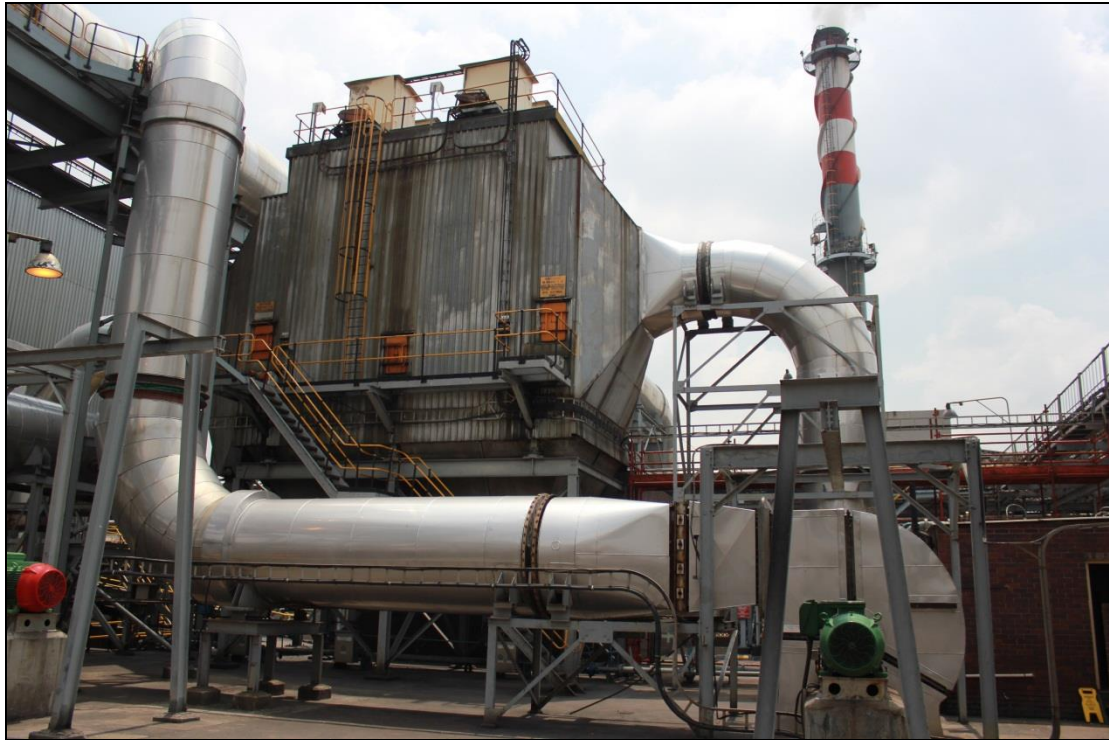
Figure H3A: Boiler ESP, ID fan and stack.
