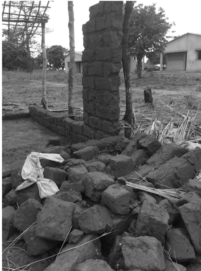
Figure 40: Picture of an unfinished Frelimo marquise in Minuco, Ribáuè, 2016
