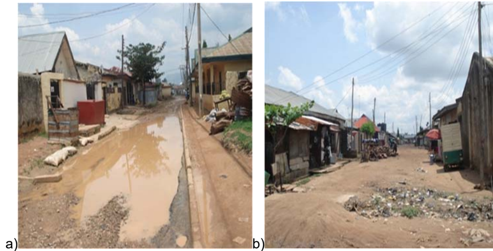
Figure 4.12 a & b: Poor road infrastructure at Karu new layout area Source: Authors fieldwork, (2017)
