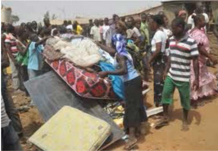
Figure 4.14: Demolition at Mpape neighbourhood Source: Vanguard Newspaper, September 25, (2012)
