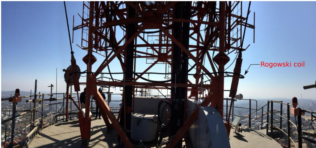
Figure 3.3: Photograph showing the installed Rogowski coil at the base of the mast on top of Sentech Tower. Within the protective tube is 2 separate coils.
