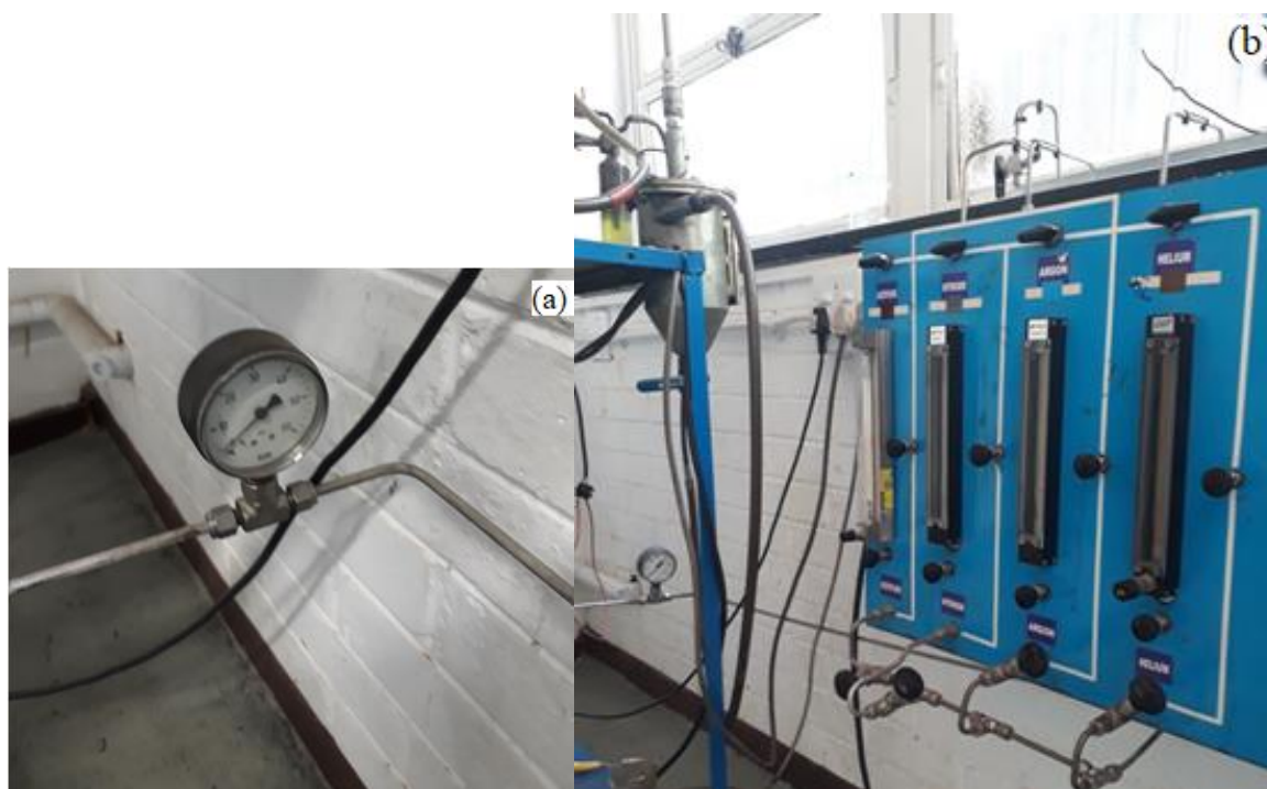
Figure A3: Control panel showing (a) pressure gauge for pressure monitoring (b) rotameter for methane gas, argon gas, and hydrogen gas channelled through to the vaporizer via a single pipe monitored by a pressure gauge.
