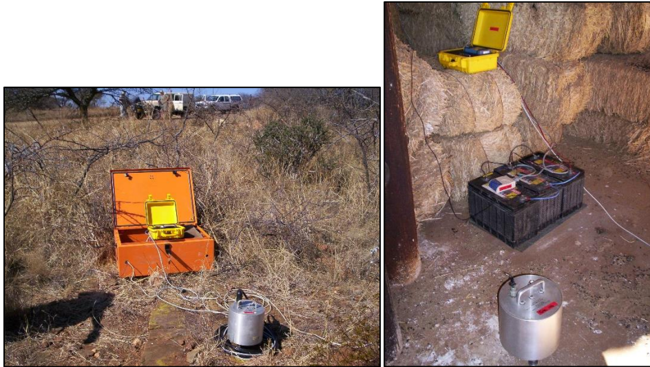
Figure 8. Typical installation of stations within the mobile network.
