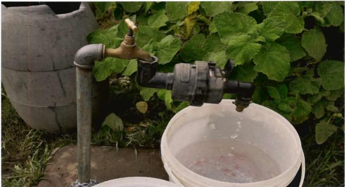
Figure 4.6: Water demand measured from a flow meter homesteads 3.
