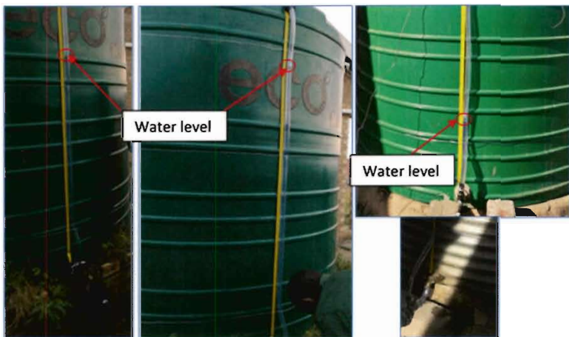
Figure 4.11: Typical storage water level measurements.
