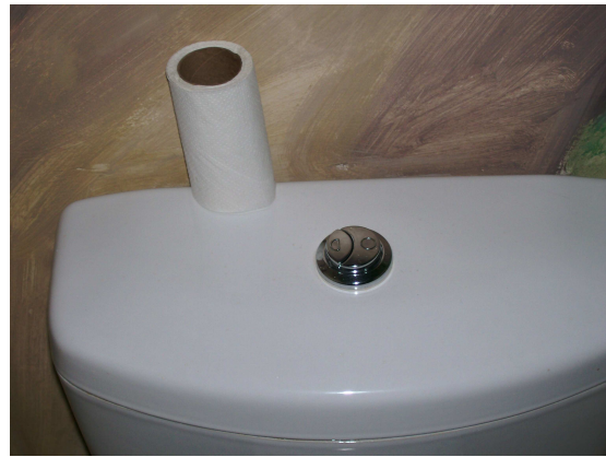
Photo 6.2: Dual flush toilet system in the centre
