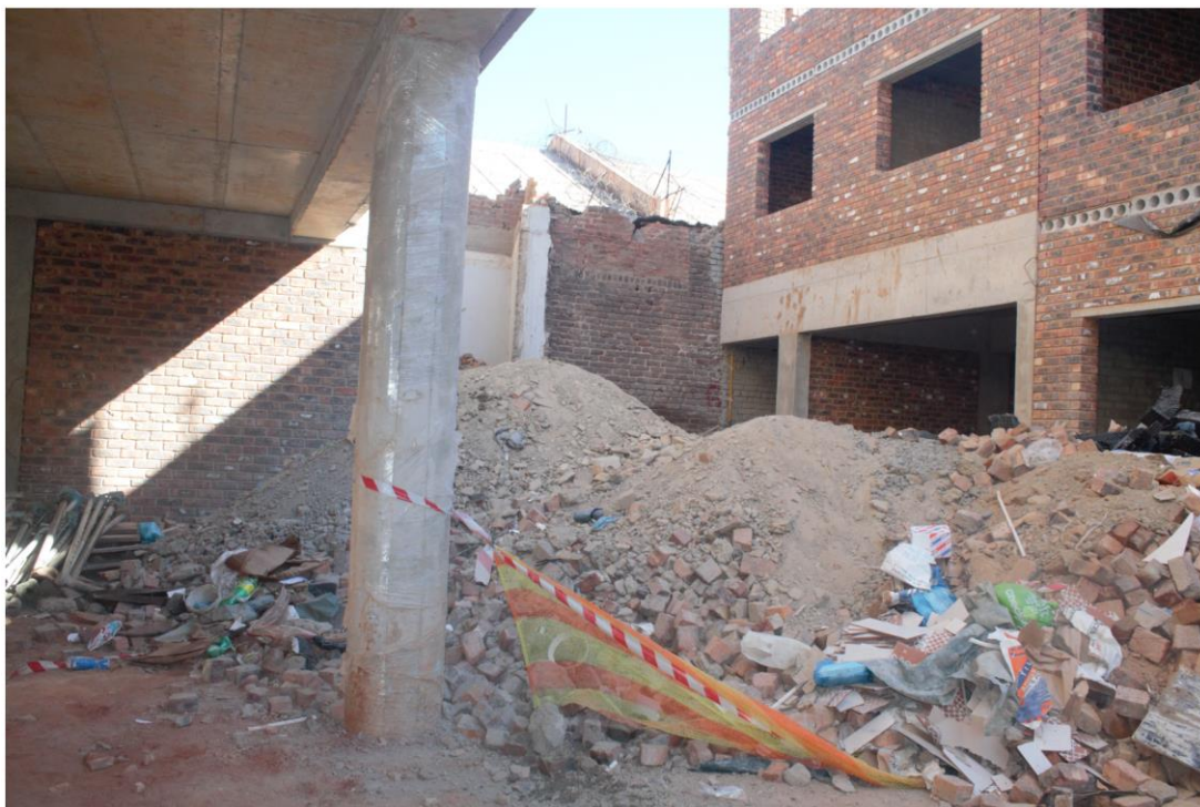
Figure 31: A view of waste material which included a mix of concrete, bricks, paper and plastic
