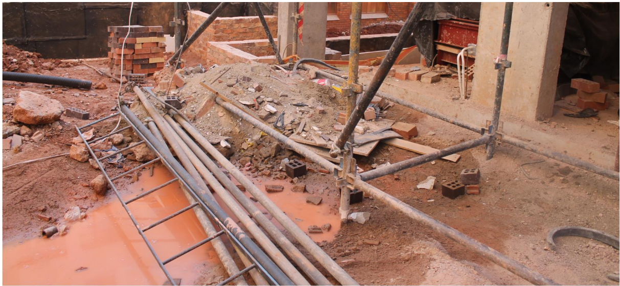
Figure 22: Waste concrete and bricks on the site during construction
