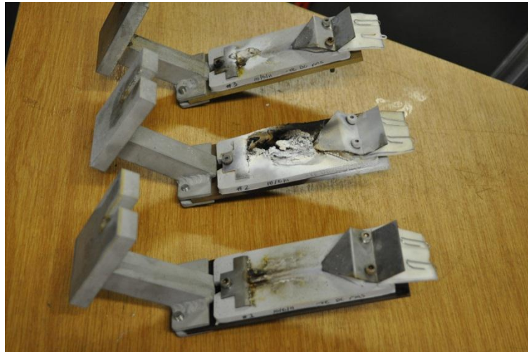
Figure C.36: DC samples showing varying stages of erosion
