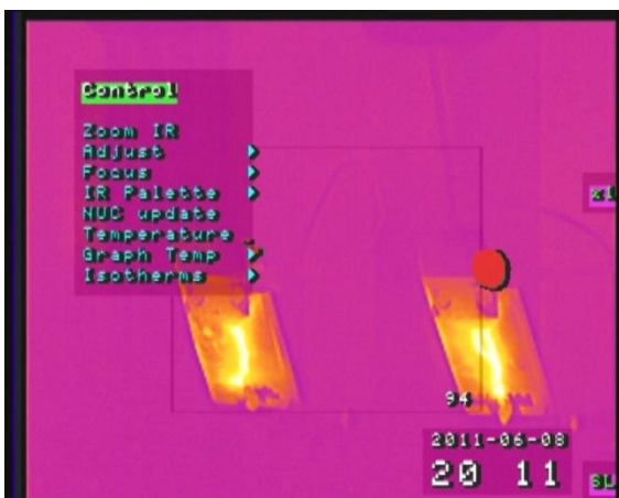
Figure C.12: IR image of leakage current
