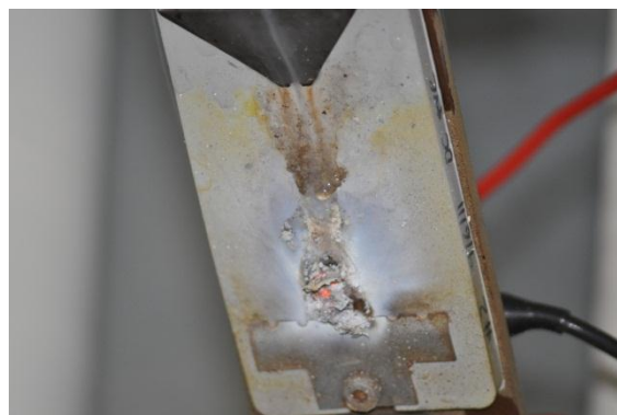
Figure C.21: Erosion at ground electrode
