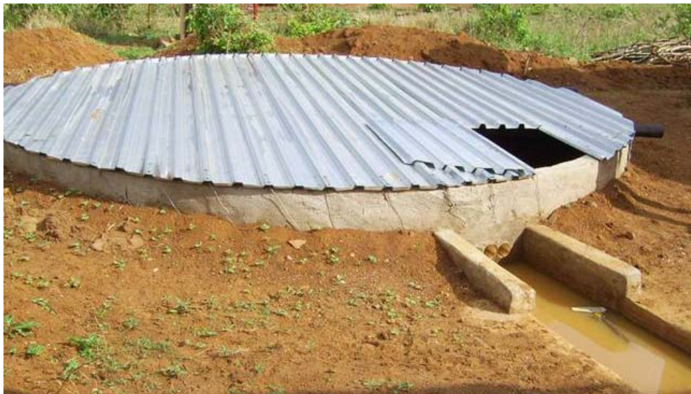
Figure 2.2. DRWH underground tank (Photo, Dams for Africa).
