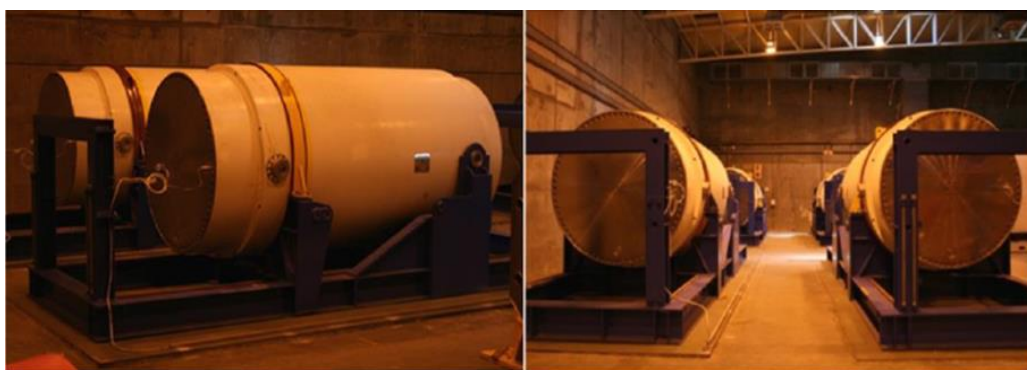
Figure 3.6: Castor X/28 casks installed horizontally at Koeberg Power Station [31].
