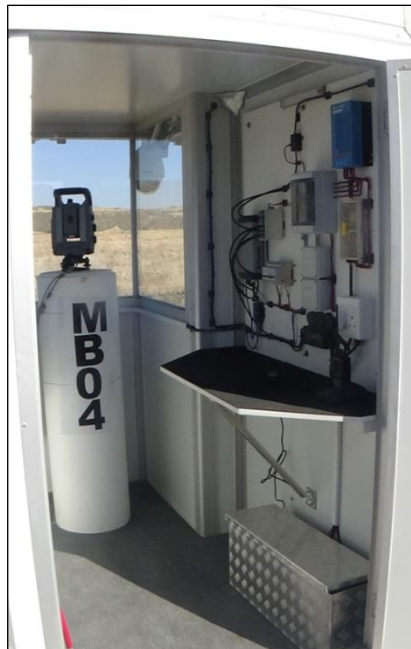
Figure 2.1: Prism monitoring station. Source: Orapa Survey Department.
