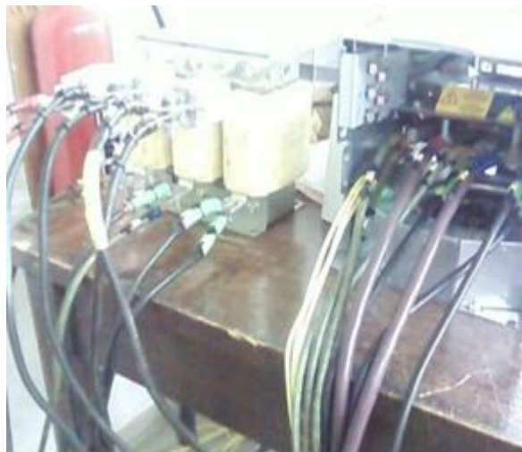
Figure 5.5: Picture of labelled DC Siemens Drive connecting to Siemens reactor and Siemens 3NE fuses
