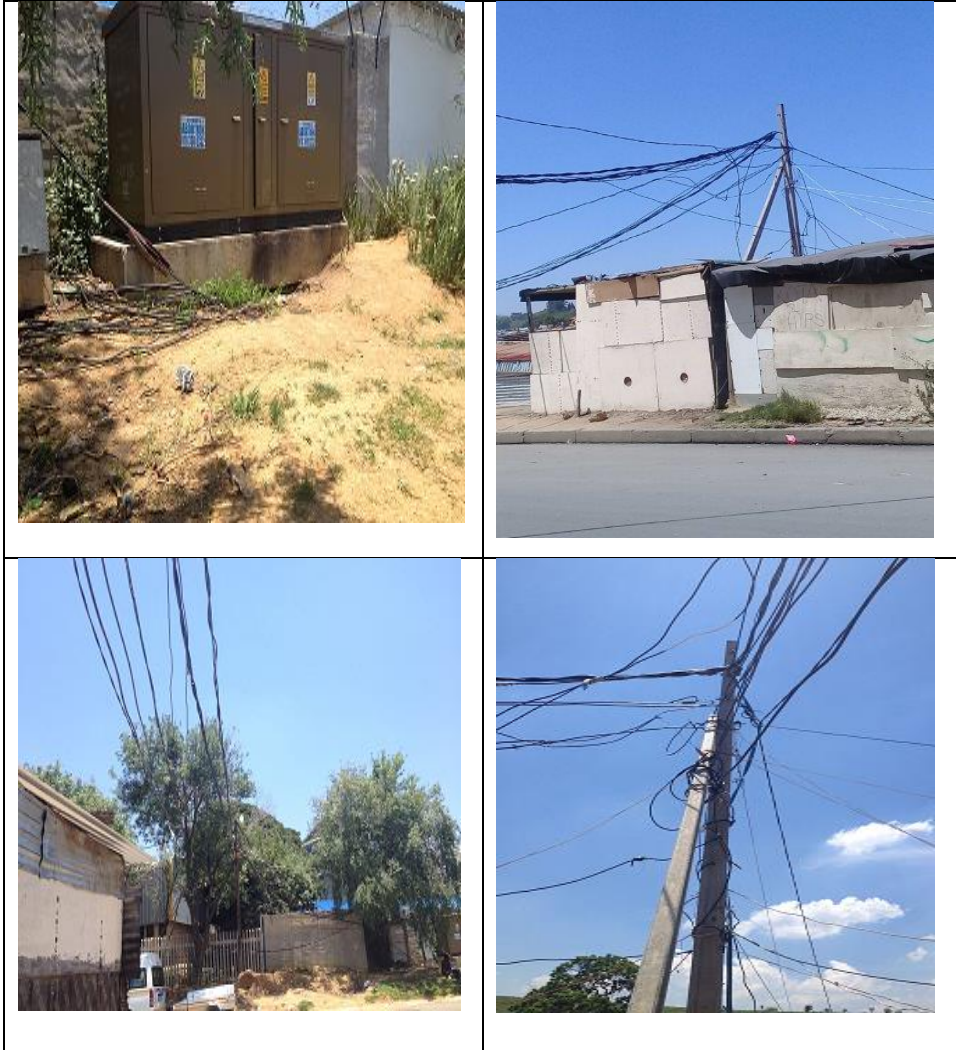
Figure 4.3: From Left to Right photo showing informal connection of electricity to Kya Sands shacks that are nearby the industrial area where the electricity is being informally connected. Source: author's own photo 24 th September 2017.
