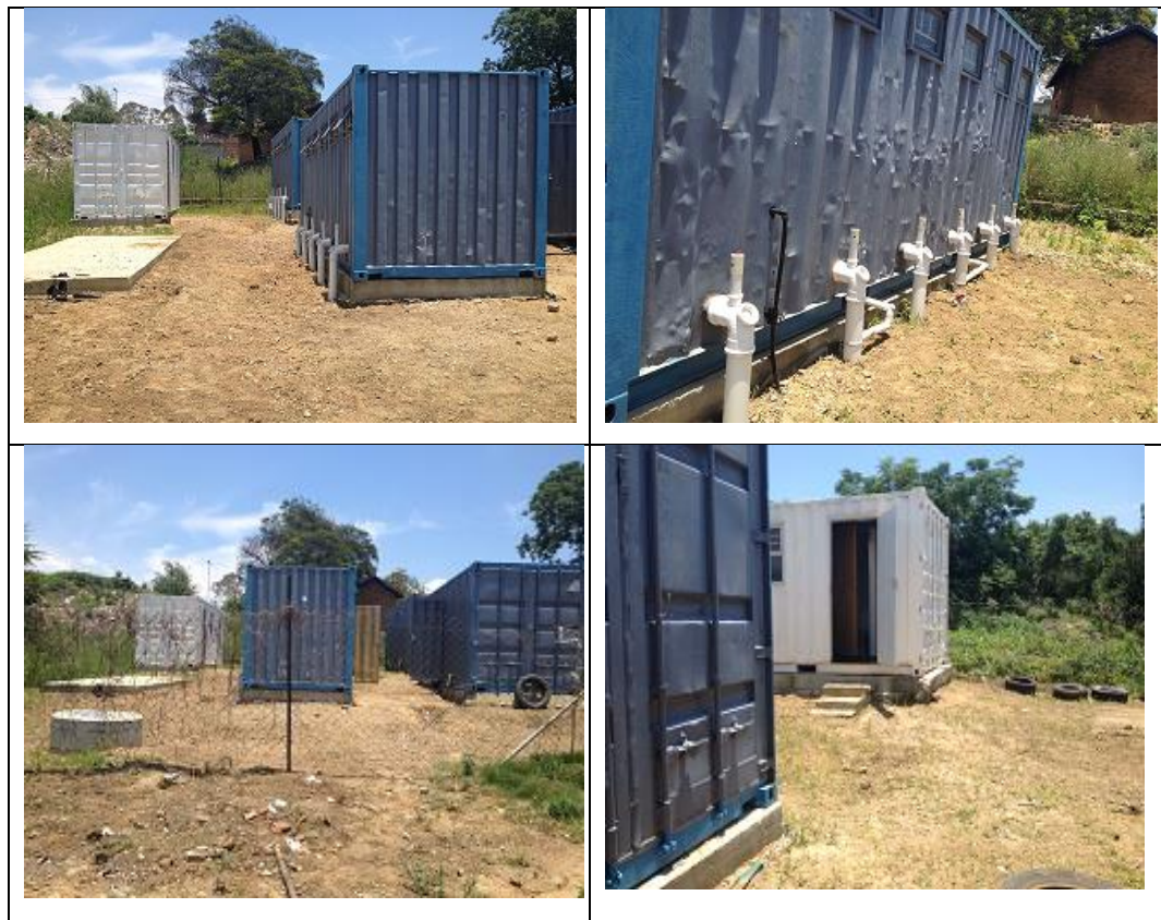
Figure 4.7: Photos showing locked, un-used flushing toilets that were built by the CoJ
