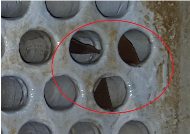
Figure 3: Condenser inside tube particulate fouling at a power station in the utility.
