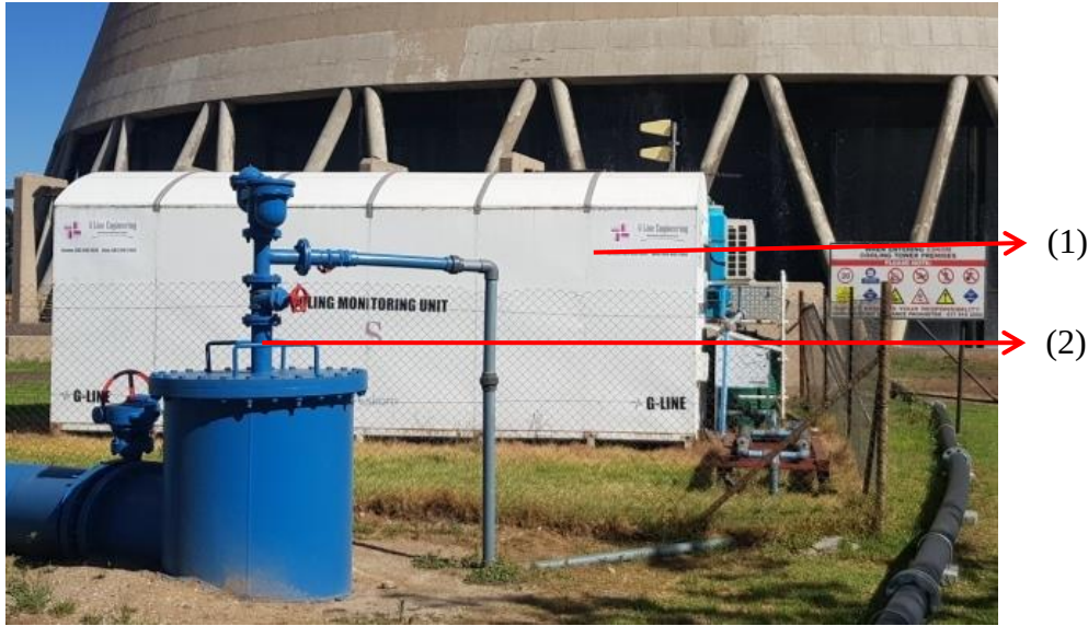
Figure 9: The location of the test apparatus on the actual plant - (1) Test apparatus, (2) 10% tap - off line
