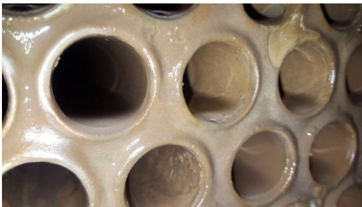
Figure 2: Condenser inside tube precipitation fouling at a power station on the utility.
