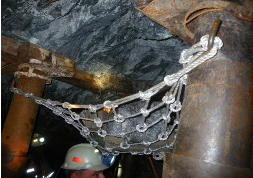
Figure 6.3.3 In-stope netting in action at Thuthukani Shaft, KDC.
