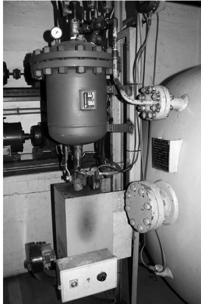
Figure 4.2: Air dryer unit
