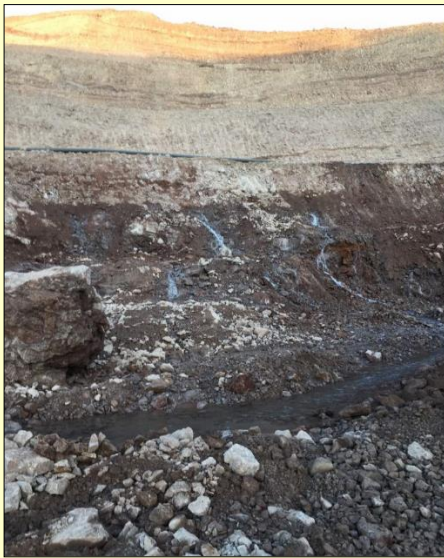
c) Seepage on the northwestern highwall in Mashi Pit.
