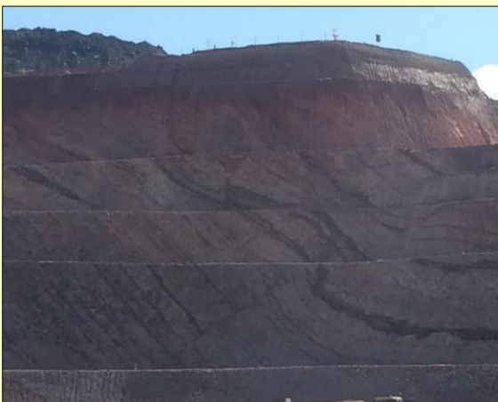
e) Folds and faults delineated by seepage (facing NW).
