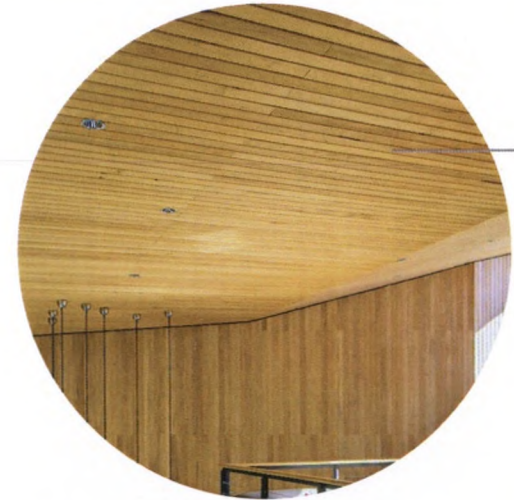
FIG 7.58: Timber acoustic treated ceilings
