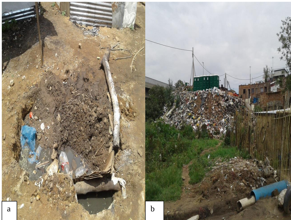
Figure 4.26: (a) failed drain design (30/01/2018) and (b) pipes draining water to Jukskei (01/02/2018).
