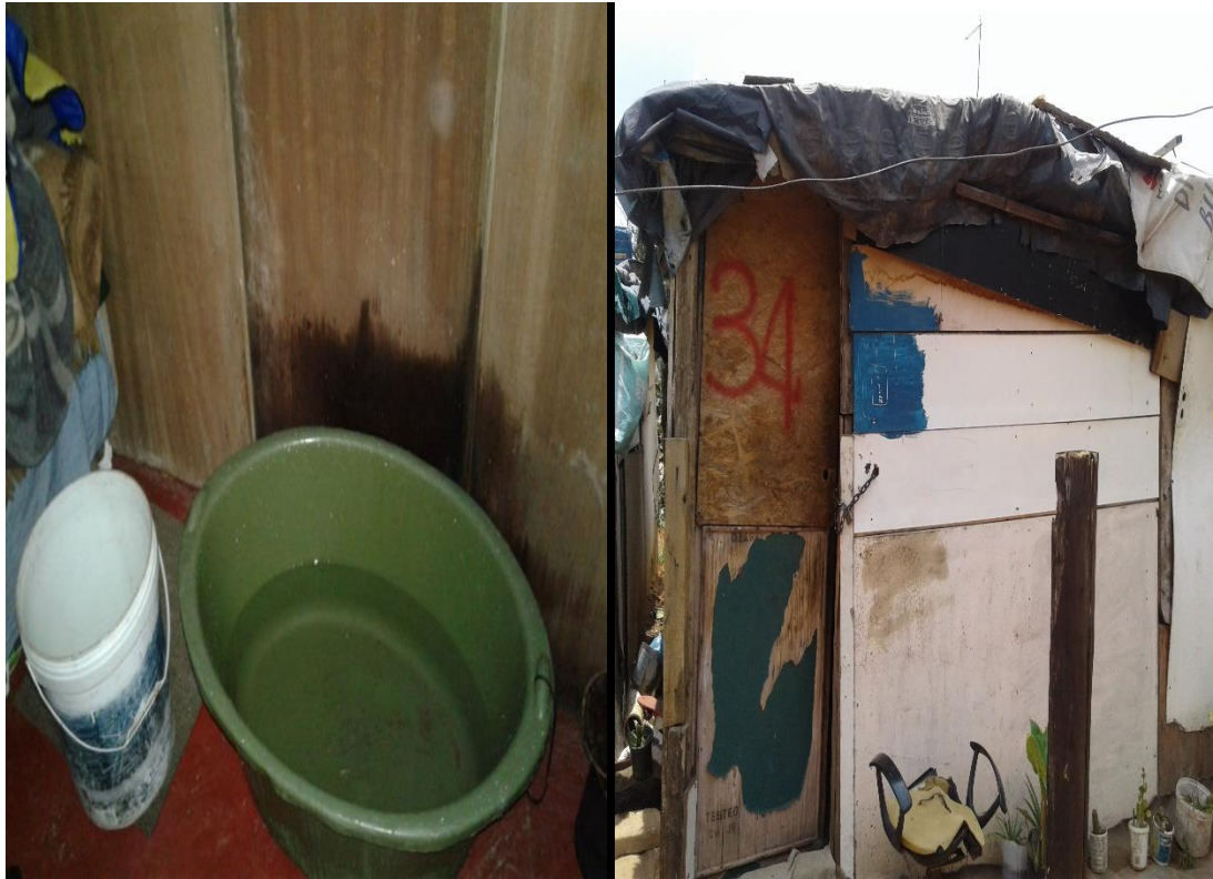
Figure 4.21: Buckets and basins used to catch water inside the shacks (23/03/18) and a plastic sail to cover the roof (30/01/2018).
