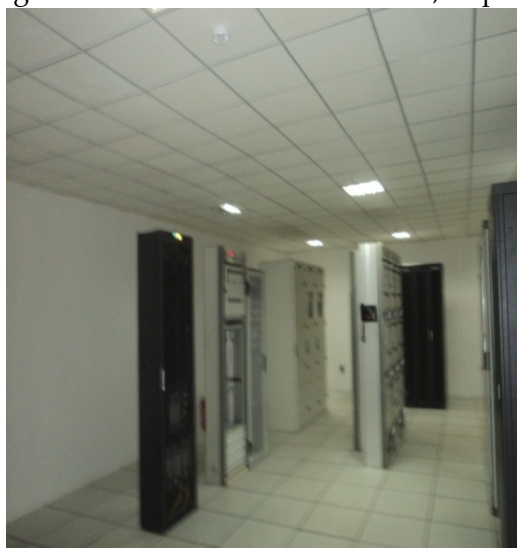
Figure 4.3 Landing station data centre at Matombi, Republic of the Congo
