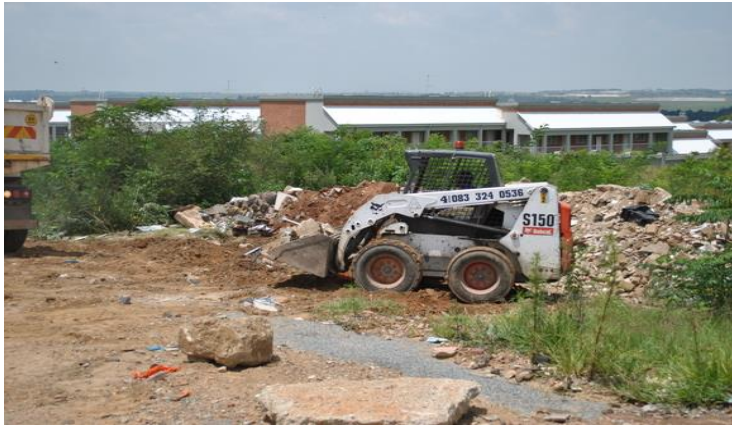
Figure 2.3: Illegal dumping of construction waste in Sandton
