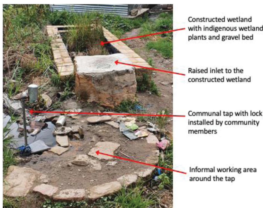
Figure 2. One of the two pilot constructed wetland systems that were installed in February 2020.
