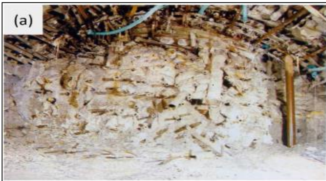
Figure 19: Bamboo piling at tunnel face at failed section (Diwakar et al. , 2022)
