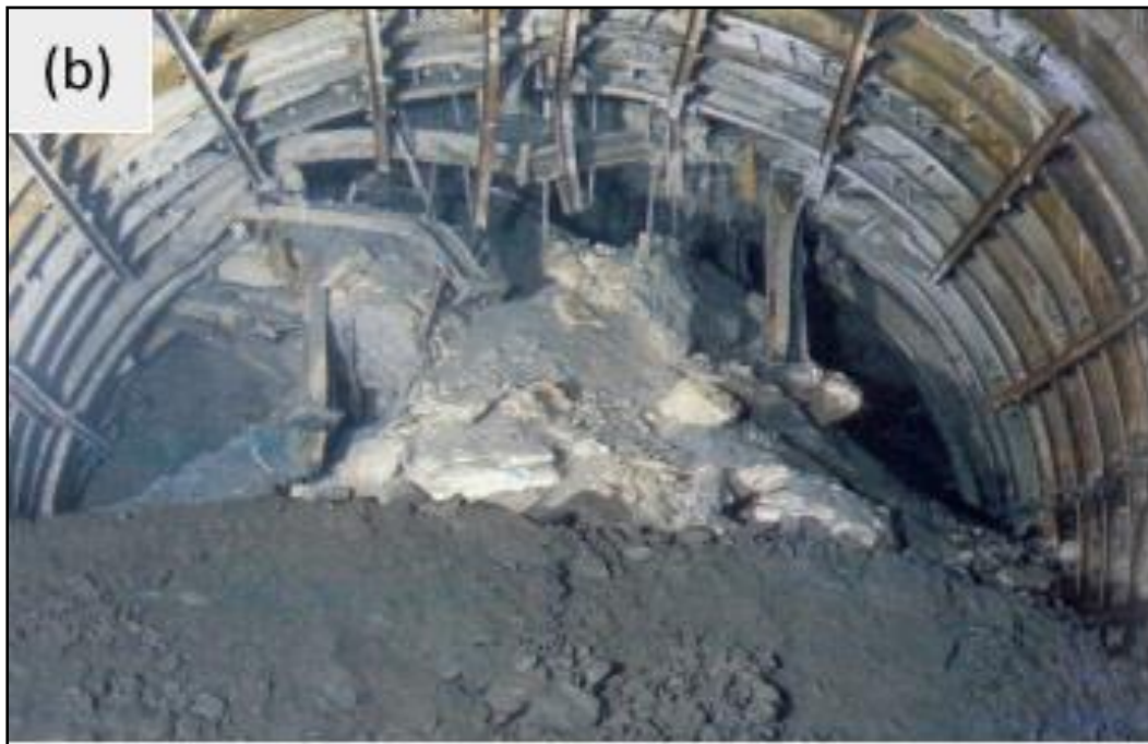
Figure 20: Failure of the ribs at the crown portion in THPS (Diwakar et al. , 2022)
