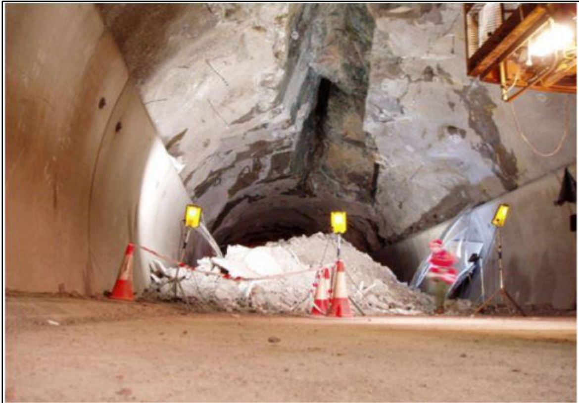
Figure 24: Collapse at the Hanekleiv tunnel in 2006 (Nihayat, 2022)
