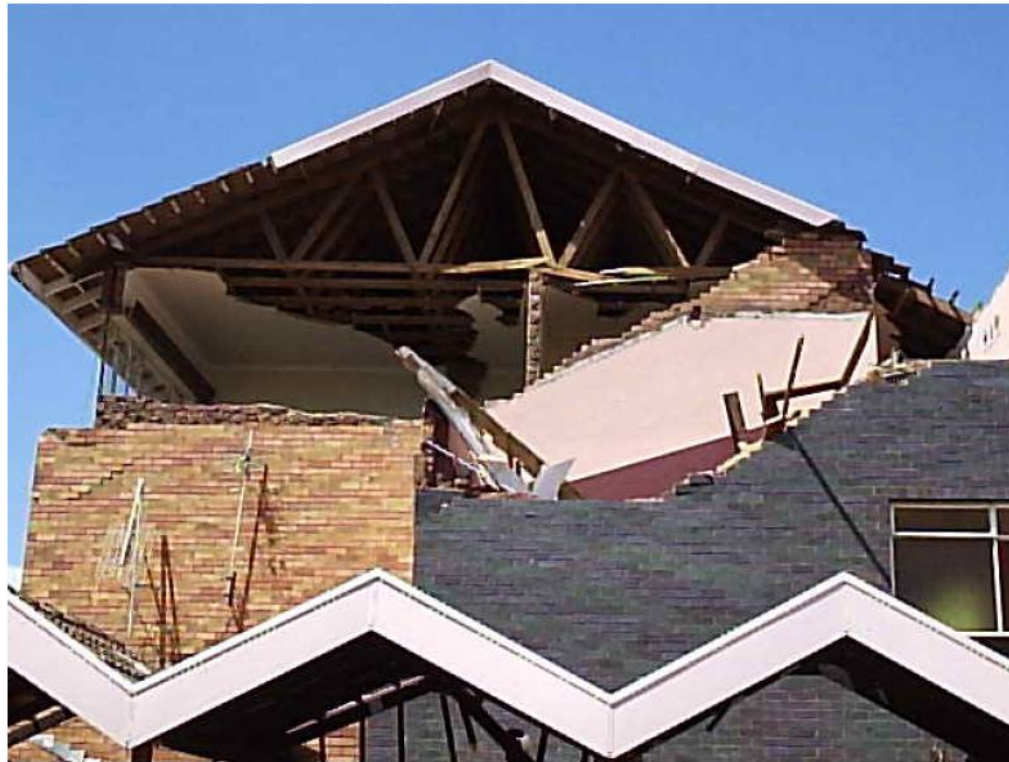
Figure 2. Structural damage observed during the Stilfontein March 2005 earthquake (Saunders et al., 2008).
