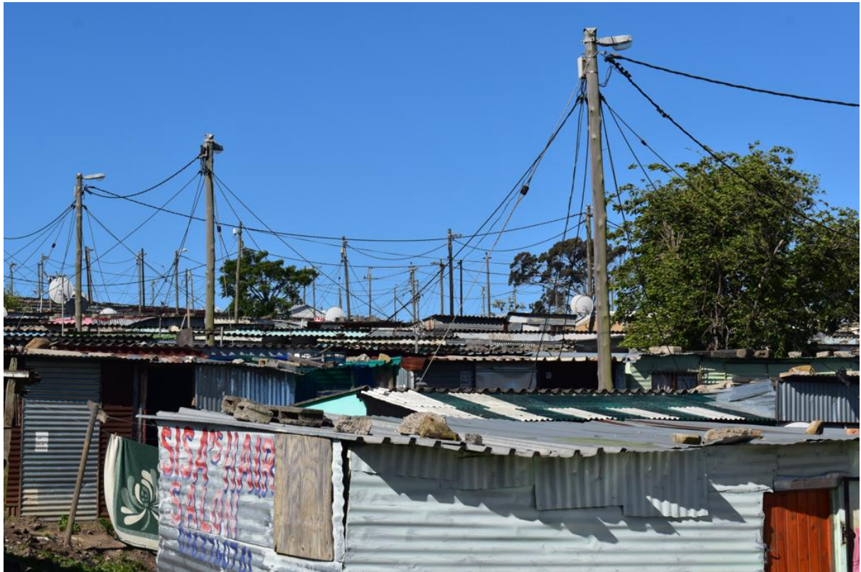
Image 33: Everyday ways of accessing electricity for those marked as informal. Where the state cannot provide, residents make means to access their fair share of democracy.
