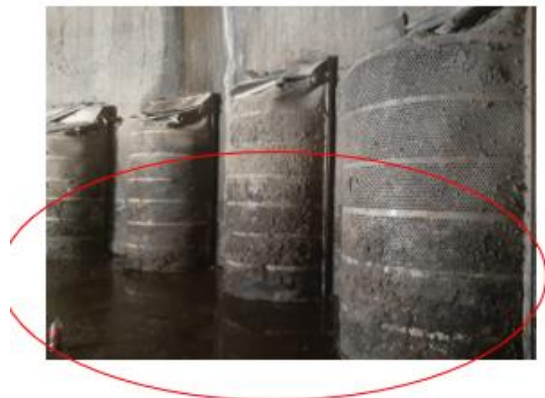
Figure 2.2.2-1: Limestone slurry buildup
