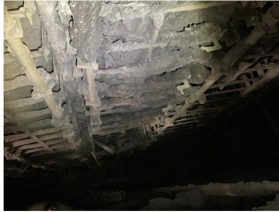
Figure 2.2.1-1: Deposits on spray headers
