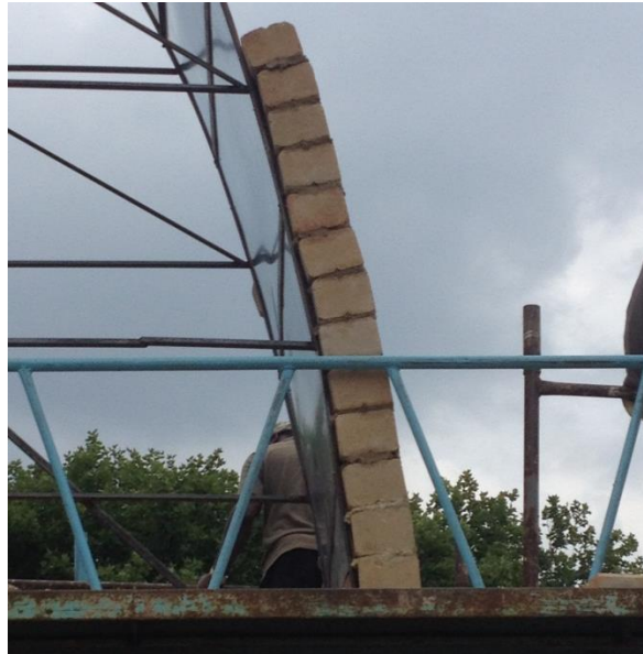
Figure 8-32: Inaccuracies in following the form during construction
