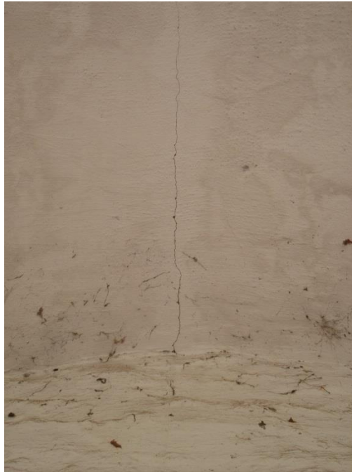
Figure 6-4: A crack occurs at the centre, or high point, of all the roof structures
