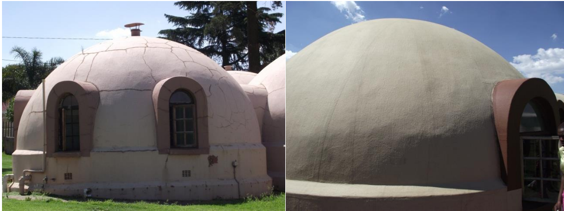
Figure 2-3: Left: A cracked dome at the Sparrow Aids Village; Right: A membrane layer is applied to the cracked dome
