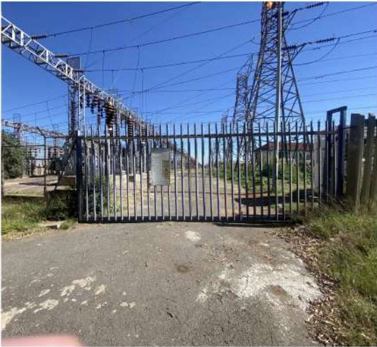
A_Restricted powerlines and transformers
