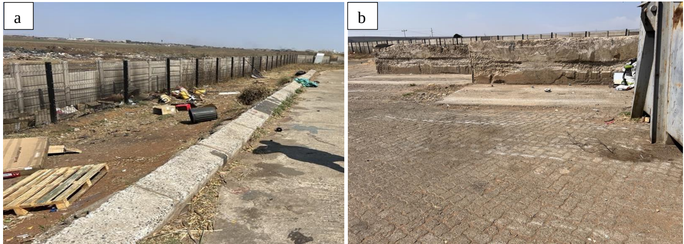
Figure 4.15a) Waste observed around the edges of the Extension 49 Waste Transfer Station b) Damage on the concrete platforms on the Extension Waste Transfer Station
