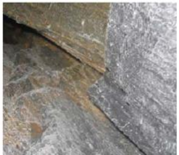
Figure 4.4.5: Phenomena of rock burst and spalling in the field (Gong, et al., 2012).
