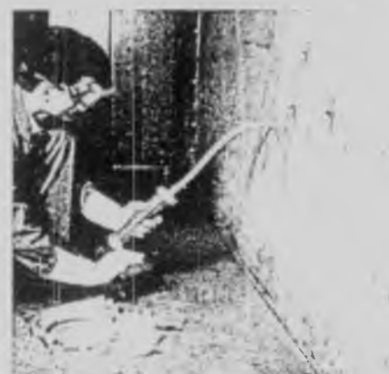
Design errors too, such as incorrect specification, or poor workmanship can affect the service life of structures. In most cases, early repair of resulting cracks is the answer.
