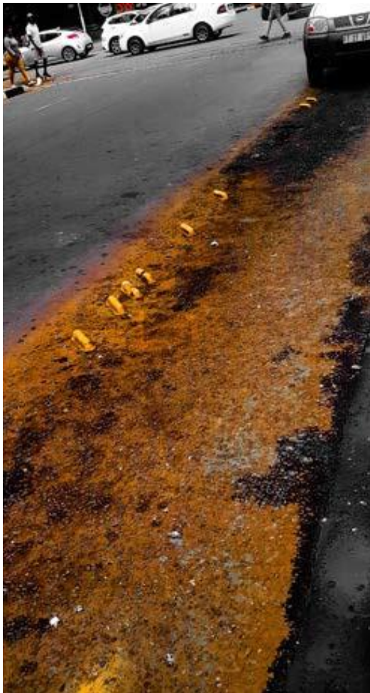
Figure 19 Damaged bike lane along Jorissen Street. Source: Author, 2023
