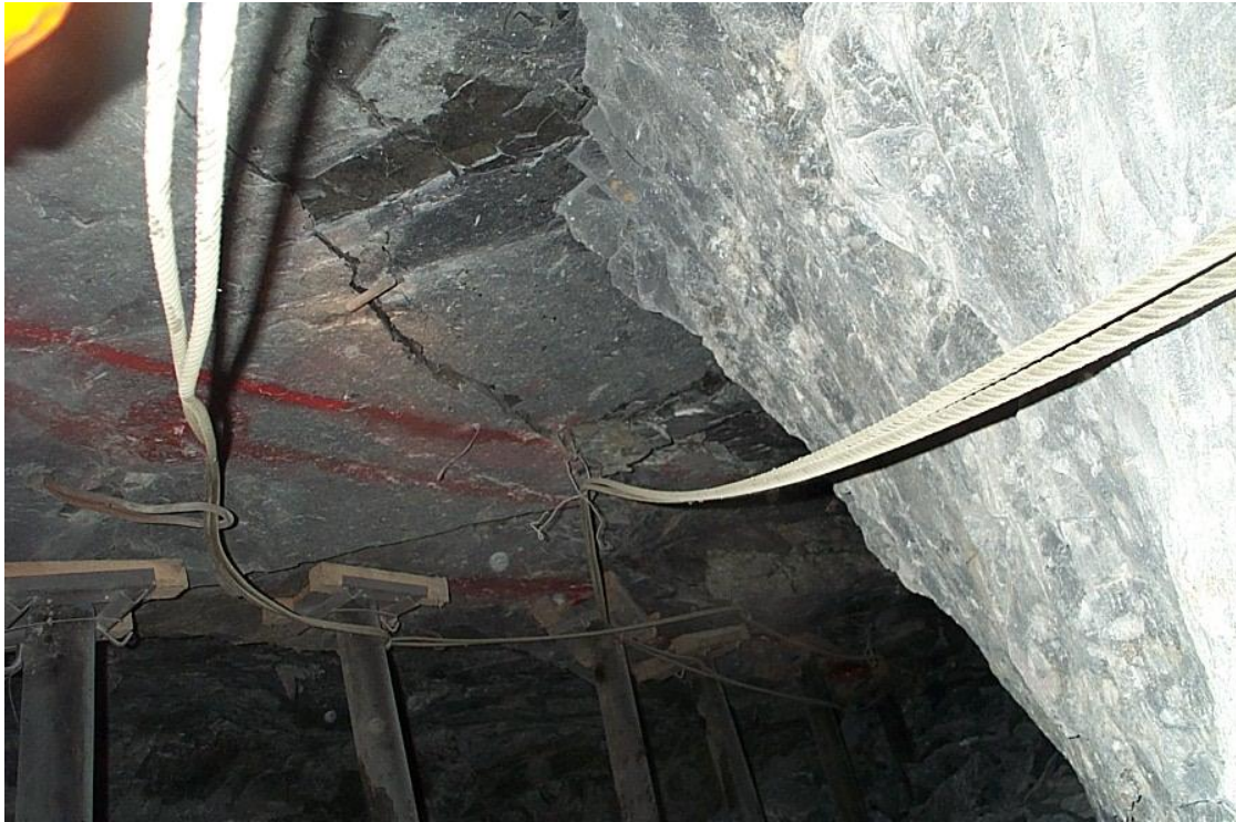
Figure 6-17 Photograph showing tensile crack failure after the ledging blast in the raise featured in figure 6-15
