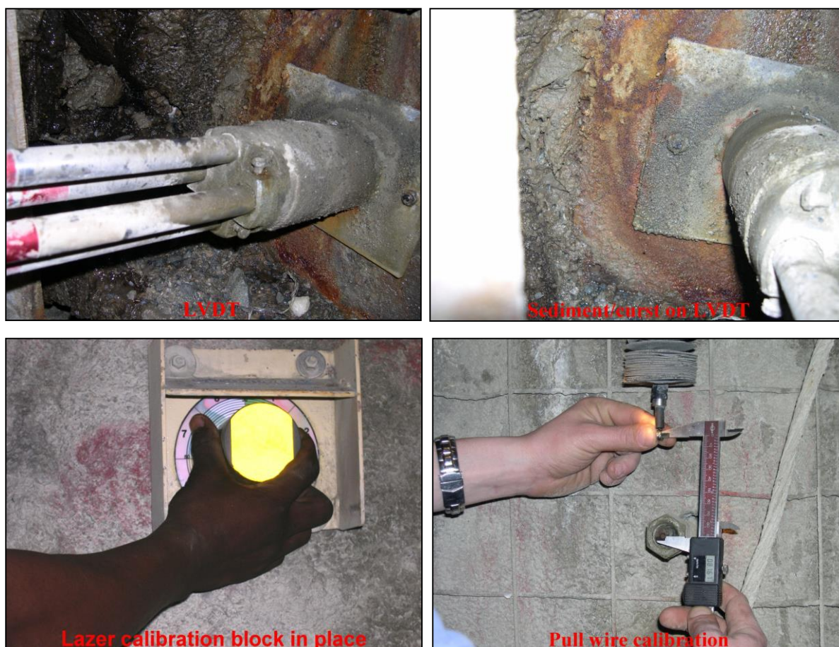
Figure 6-2 Collage of photographs (from left – multipoint rod extensometer, calcification of rod extensometer, laser sight, wire extensometer) showing the geotechnical monitoring instruments installed at Ya Rona shaft
