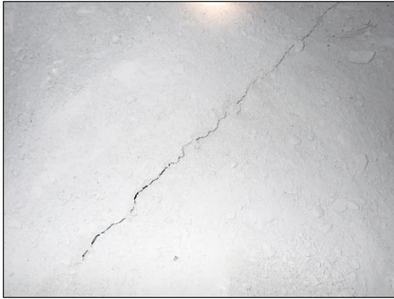
Figure 4.8: Tensile cracks in the footwall.
