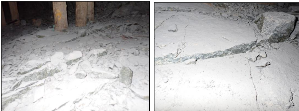
Figure 4.7: Footwall fracturing and heave around a crush pillar footwall.
