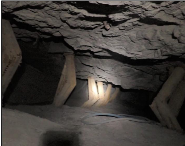
Figure 1.4: Failed mine poles in the back area of stopes.
