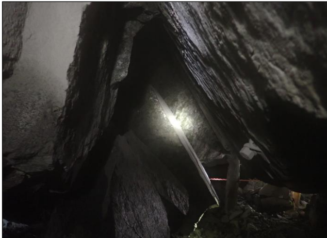
Figure 2.13: Wedge failure between joint sets.
