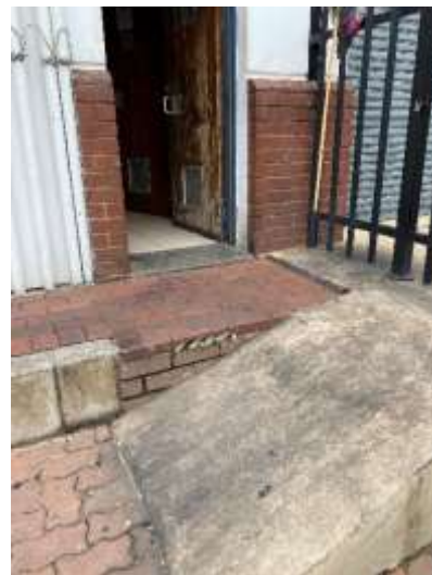
Figure 4.6 an inaccessible ramp participant 5 needed assistance to use when entering and exiting the bathroom at a petrol station
