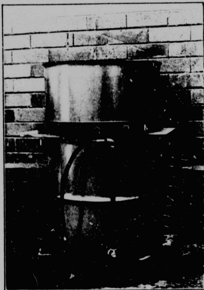
A SMALL SCALE RURAL WATER TREATMENT PLANT
