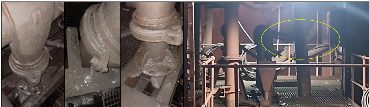
Figure 1.3: Typical single line densifier failures observed at the drum plant
