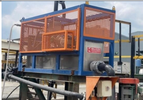
Belt Magnet and piping.
