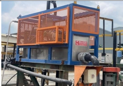
Belt Magnet and piping.
