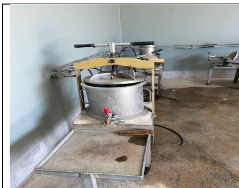
Pneumatic filter pot for filtration
