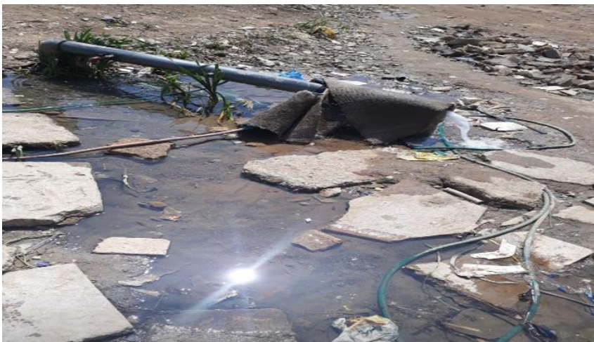
Figure 4: A standpipe that is leaking and does not close (Rangata, 2018)
