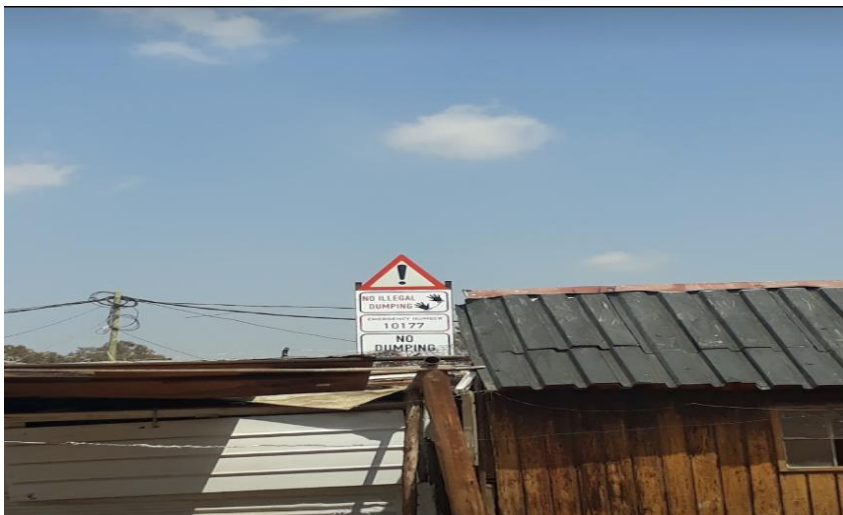
Figure 9: Illegal electricity connections hanging above a shack (Rangata, 2018)
