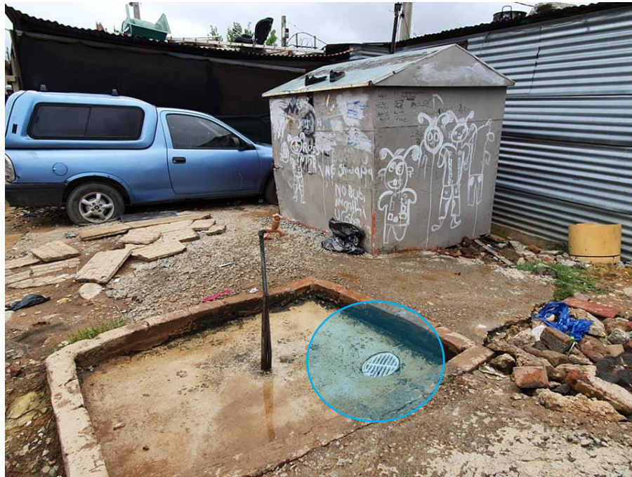
Figure 25: Drains adjacent to a communal tap.
