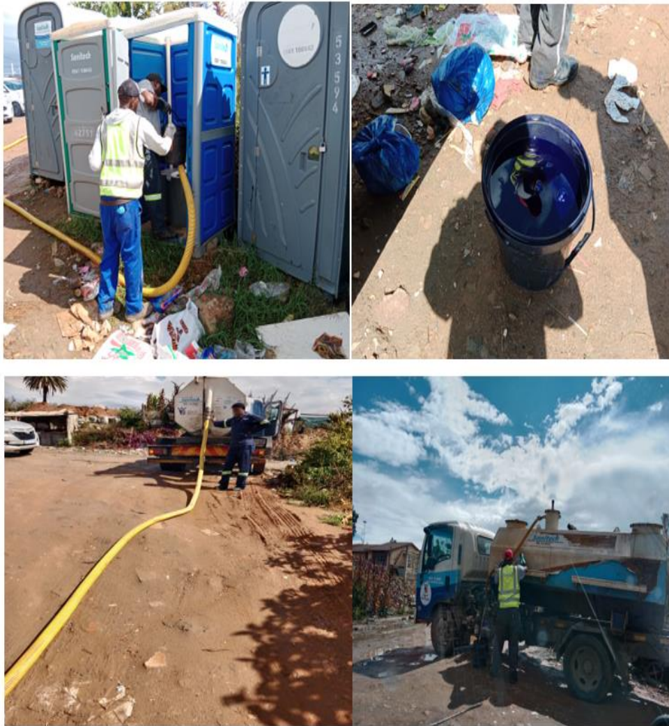
Figure 19: A sequence of toilets drained in Silvertown.
