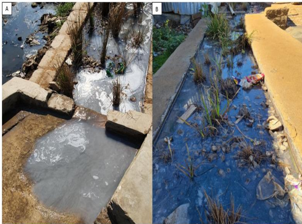
Figure 39: Flooded CW2 (A) and Flooded CW1 (B)
