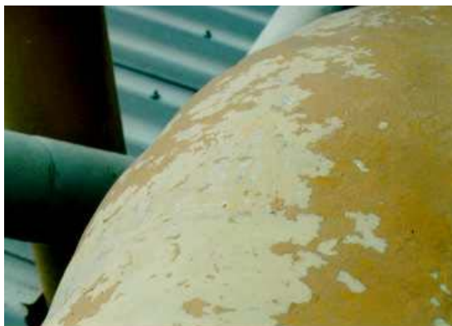
Figure 2.2 Degradation due to UV rays identified as discoloration or flaking of the surface on the topside of a pipe (with the permission of SASOL)
