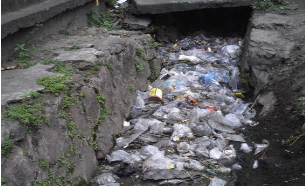
Figure 13: Untreated Drainage Channel in the corner Mbomu and Bokasa; July 2009
