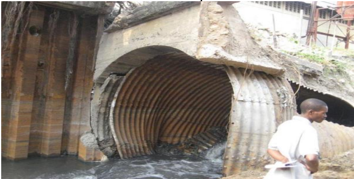
Figure 16: Blocked Drainage Channels at Bitshaku-Tshaku River Next to 24 November Stadium In the eastern part of KLM
