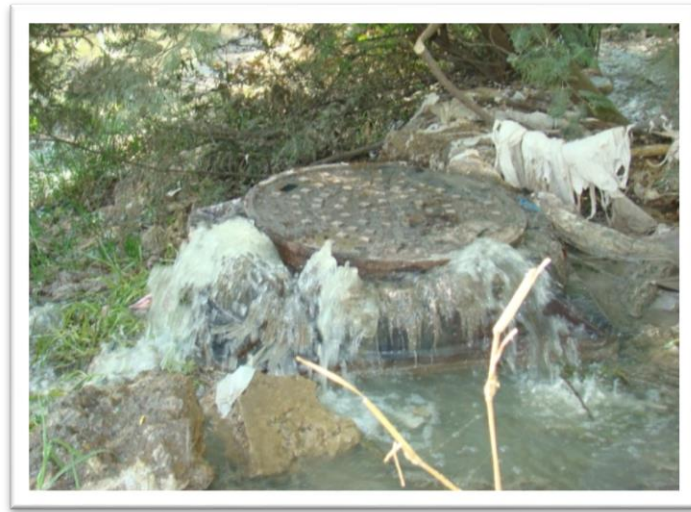
Figure 5.3 One of nine overflowing sewerage manholes prior to the Bicycle Park (Author: 2008)
