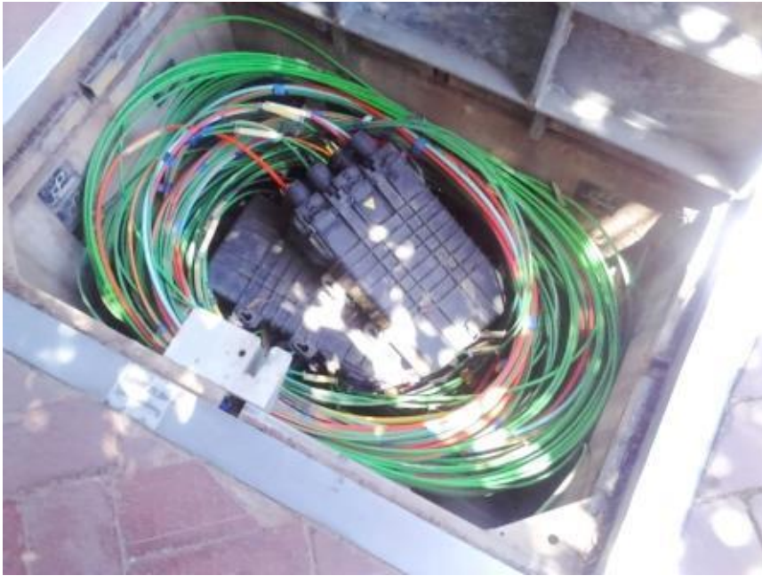
Figure 10: View under a service cover in Sandton central, Maude Street.
