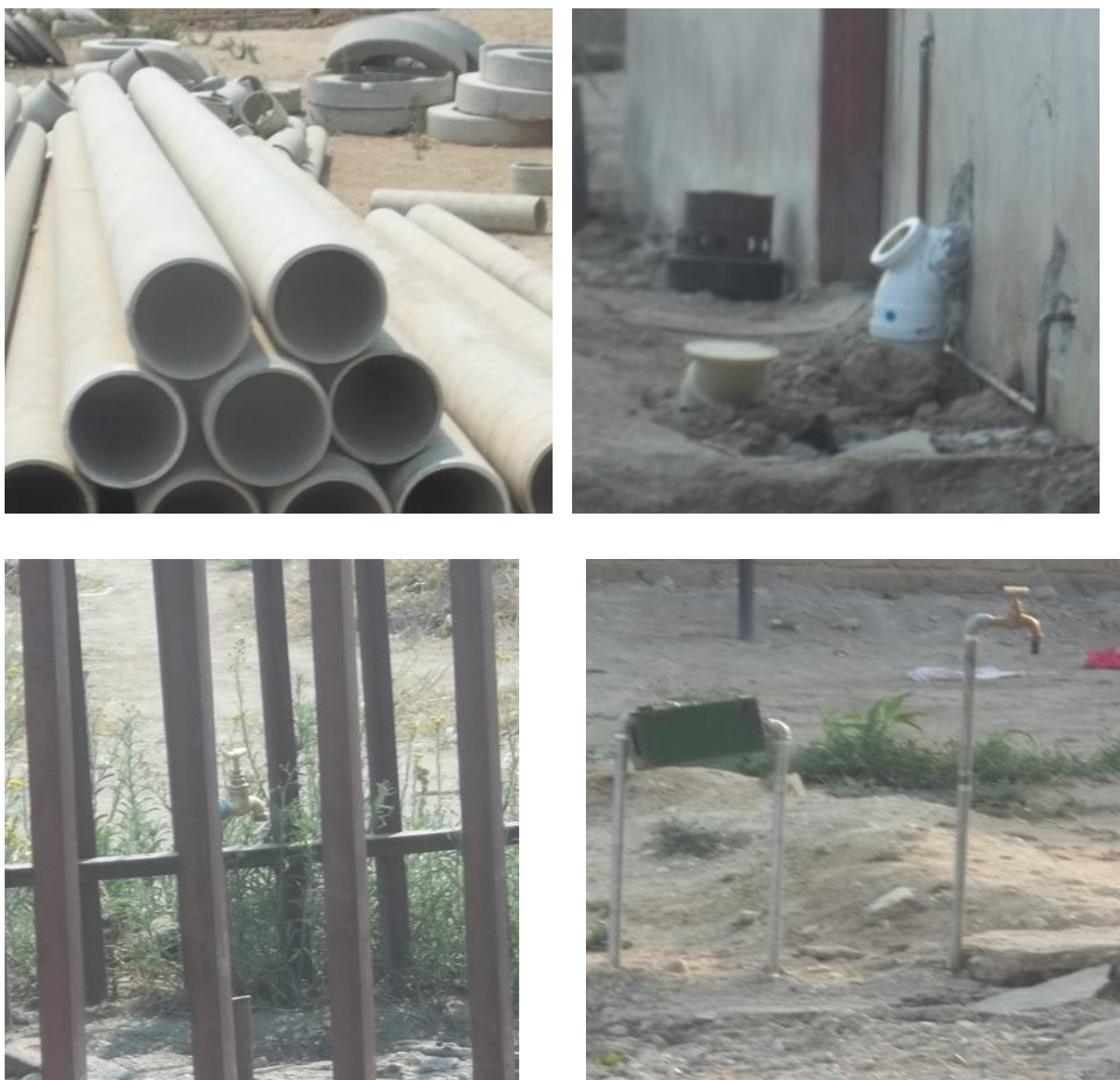
Figure 4.1 sewer pipes and water taps (authors own photographs)
